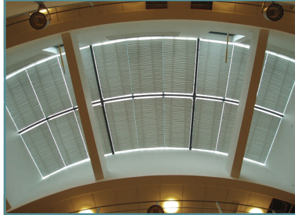
Roof louvre blinds in closed position
