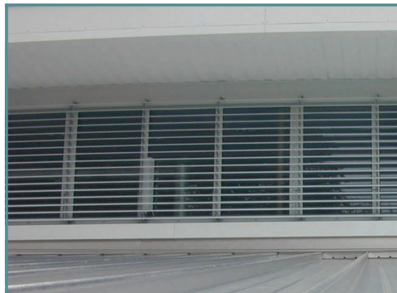
External louvres in open position
