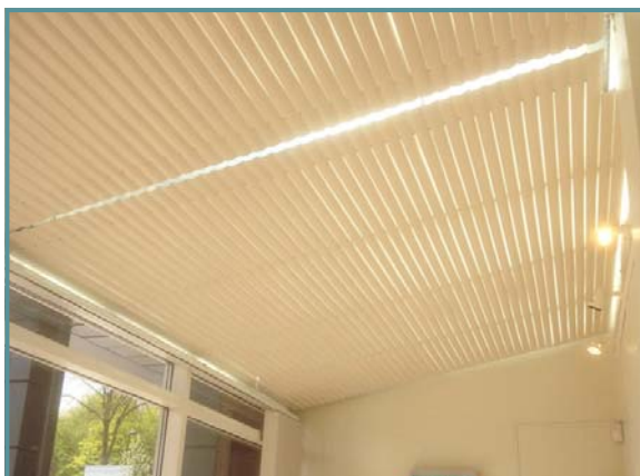
Louvre Roof Blinds Closed
