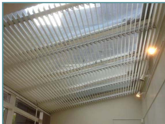
Louvre Roof Blinds Open
