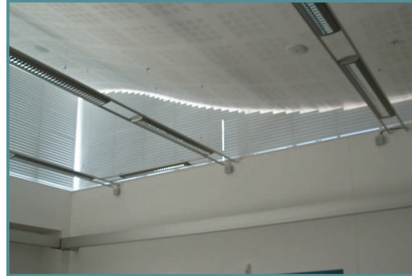
Blinds fully deployed
