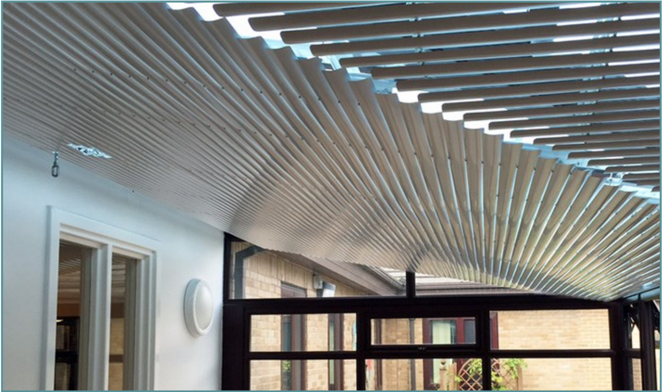
Cut-out in run of louvres to accommodate the window actuator mechanism
