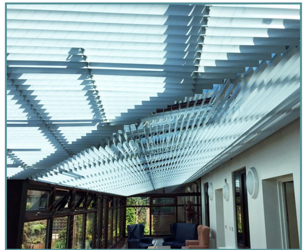
Louvres in fully open position
